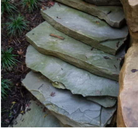
Detail of green biological growth on hardscape.
