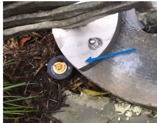
Detail of sprinkler head next to the sculpture.
