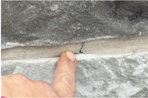
Detail of cracks in grout.
