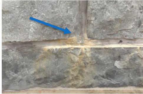
Detail of possible efflorescence on walls.
