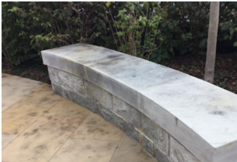
Detail of tannin staining on floor pavers.
