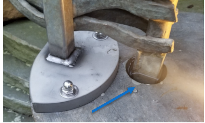
Detail water standing in concrete bases.
